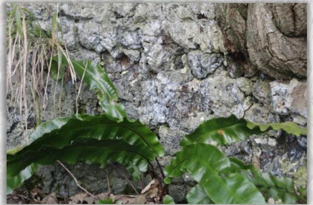
Fire damaged stone in the Kiln
